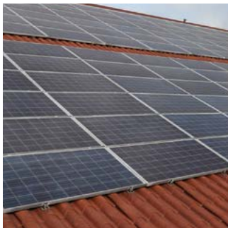
Use of renewable energies: photovoltaic panels
